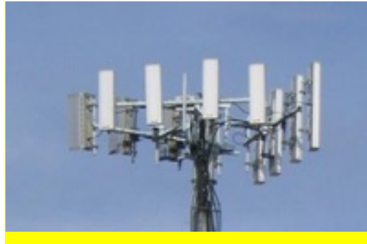
Traditional Cellular Antenna
